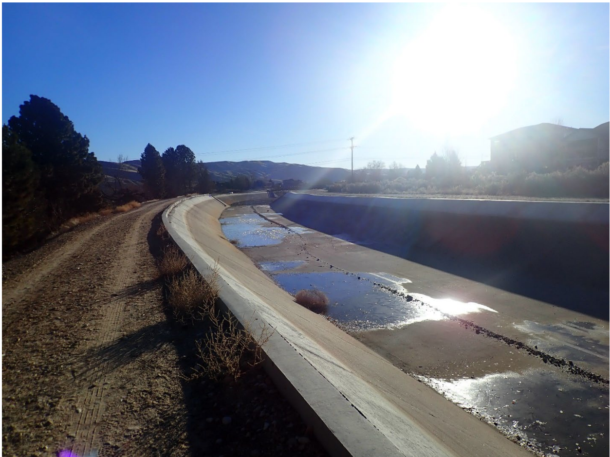
Figure 11. A stretch of the New York Canal during a period when it has been dewatered. The photograph shows the adjacent gravel access road. This location is just east of where the proposed lining would begin. This view is facing east and shows a segment of canal where lining has already been installed.
